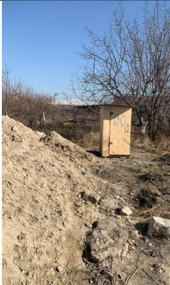
Sanitation place availability in construction site, Lenughi MA/ Lilanarm LLC/
