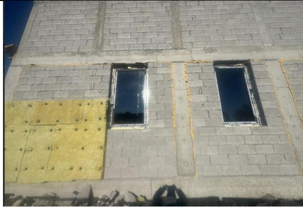
Thermal insulation of walls (Vardanashen MA)/ Kankarshin LLC and Art Plast LLC/
