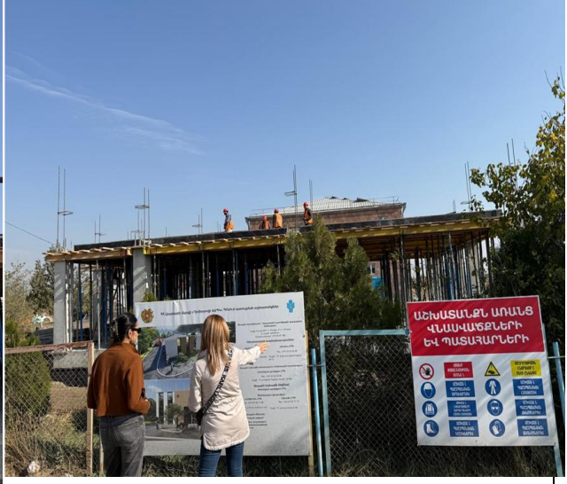
Visit of ADB representatives to the Dimitrov MA construction site /Shahart LLC and Blesk LLC Consortium/
