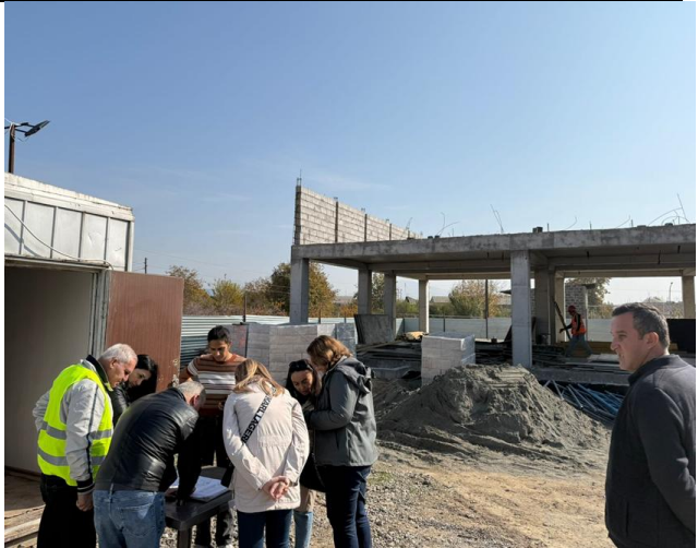
Project design discussion at the Aygestan MA construction site during the ADB mission/ Shahart LLC and Blesk LLC Consortium/
