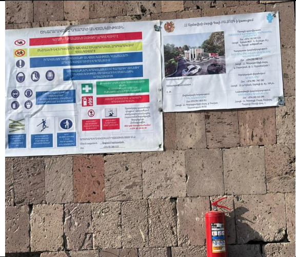
Information board, warning signs and fire extinguisher are installed(Gay MA)/ Ela Shin LLC and Lilanarm LLC/
