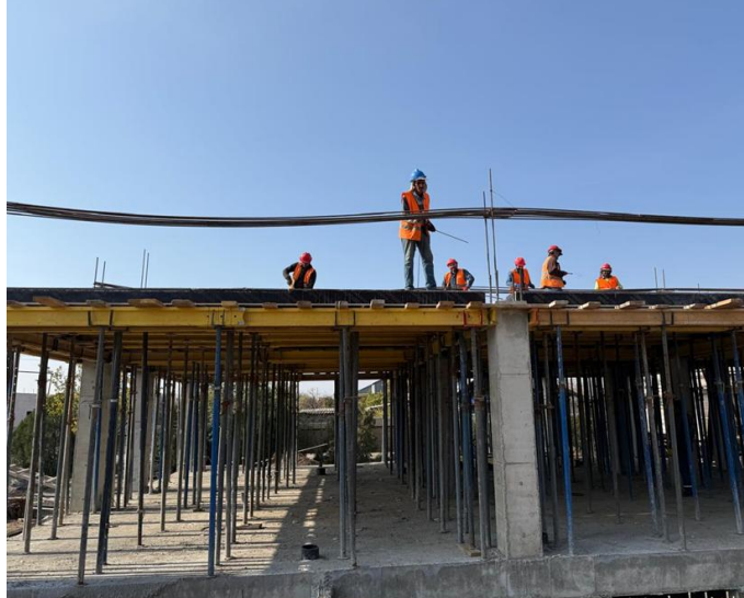
Personal protective equipment, Dimitrov MA construction site /Shahart LLC and Blesk LLC Consortium/
