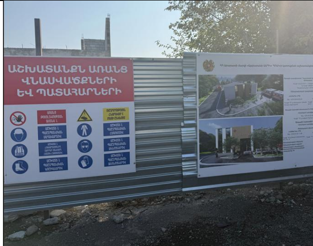
Information board and warning signs are installed(Aygestan MA)/ Shahart LLC and Blesk LLC Consortium/
